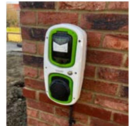
Electrical Vehicle charging point at Coppers Lane, Matfield
